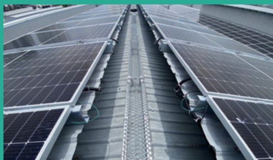
Solar panels for self-use
